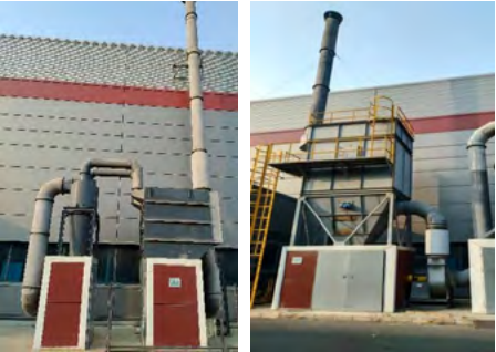
Waste Gas Treatment Equipment
