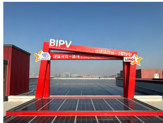
Rooftop PV System at Headquarters Office Building
