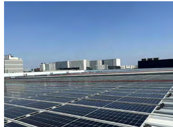
Rooftop PV System at Production Base
