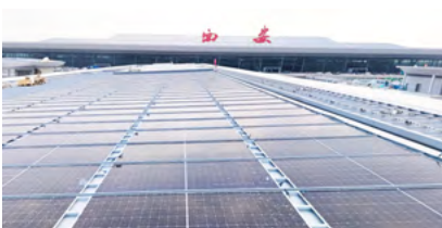
BIPV at Xi'an Xianyang International Airport
